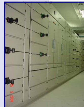
Switchgear and Switchboard
