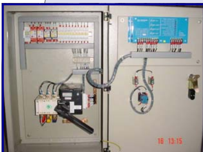
Internal View of a Transfer Switch
