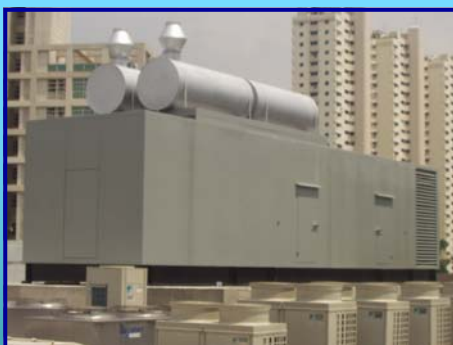
2000kVA generator sets covered with 75dBA @ 1 m Sound Proof Enclosure
