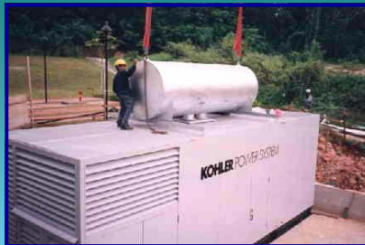
1500kVA KOHLER generator set with EN-SYST 85dBA @ 1m Sound Proof Enclosure
