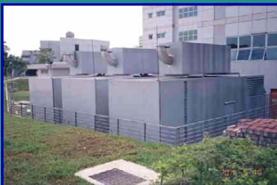
3 x 1500kVA generator sets with 85dBA @ 1m Sound Proof Enclosure
